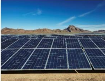
Copper Mountain Solar – Located in New Mexico
