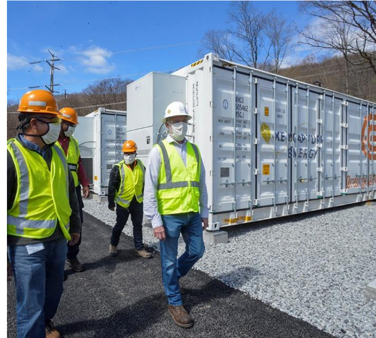
O&R's President and CEO Robert Sanchez, left, joins a walk-through of O&R's new battery storage facility. In addition to Sanchez, from left: VP Operations Orville Cocking, Project Manager MD Sakib and COO/Co-Founder of Key Capture Energy Dan Fitzgerald
