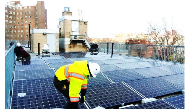
Workers installing solar panels at Carver Houses, a New York City Housing Authority development in northern Manhattan. Photo credit: Accord Power Inc.
