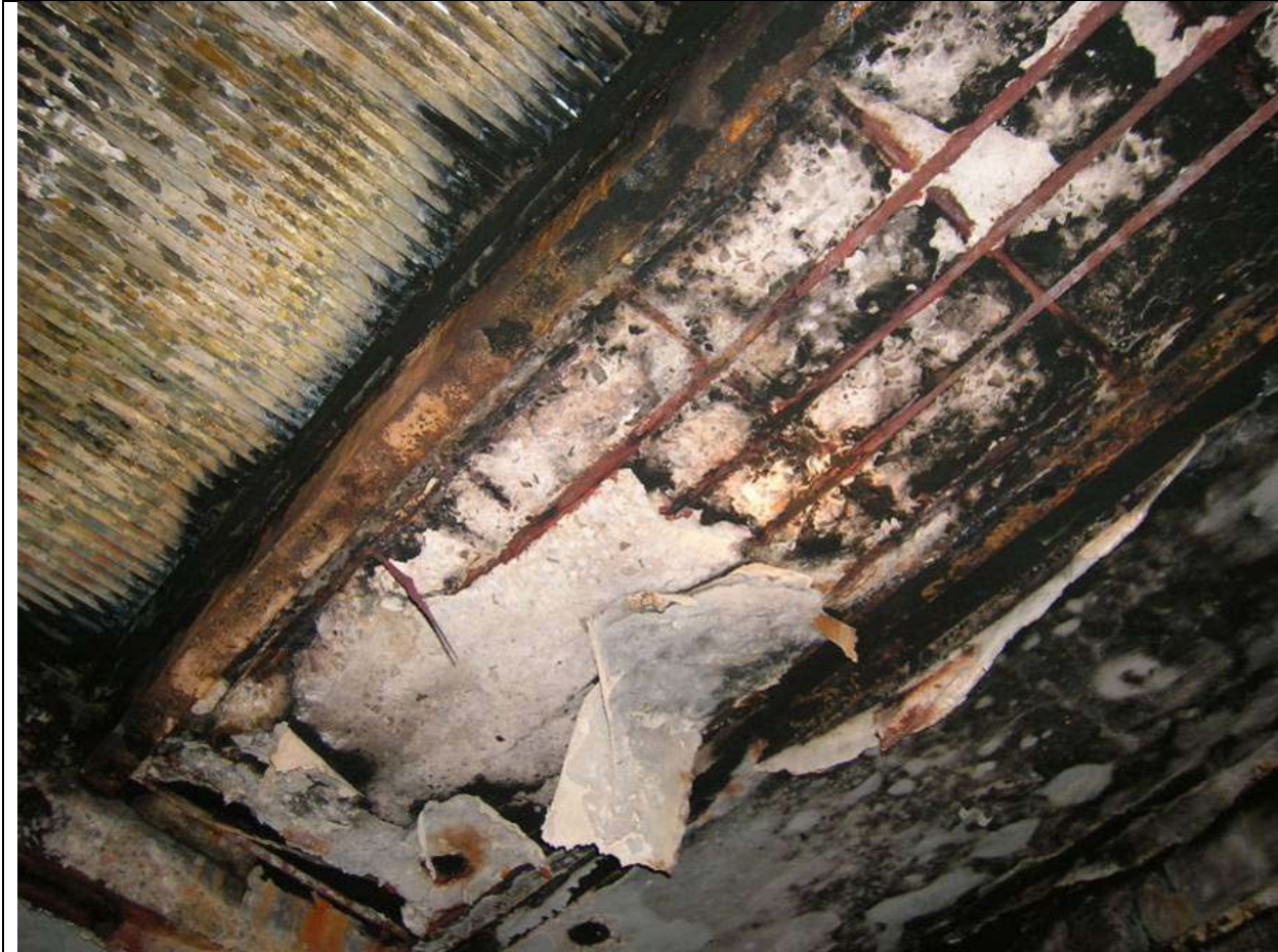
Figure 3: Delaminated concrete and debonding rebars - rood replacement is required
