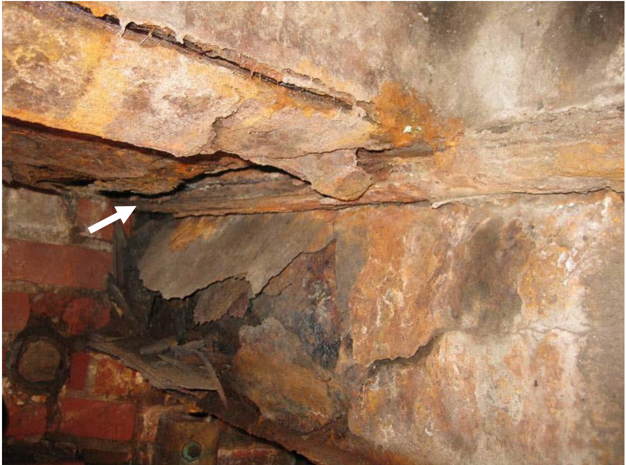
Corroded steel beam flaking at beam seat
