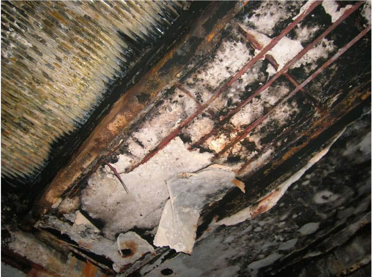
Delaminated concrete with exposed rebar – roof replacement is required (cannot be repaired)
