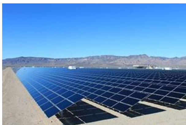
Photo above is section of Copper Mountain Solar facility in Nevada
